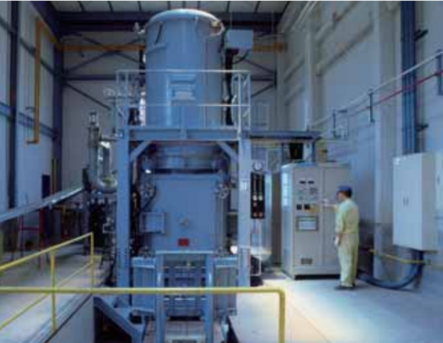
真空焼鈍炉 VACUUM ANNEALING FURNACE
